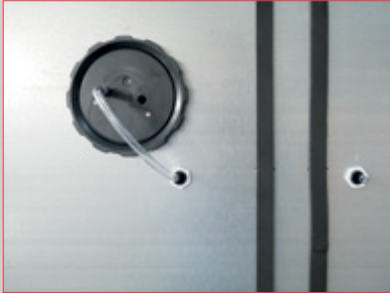
Manometer tubing within the door
