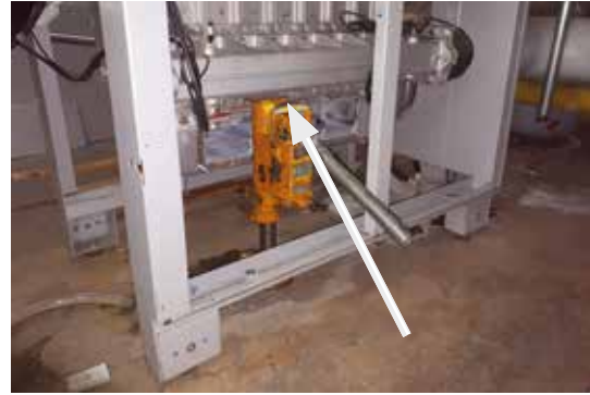
Jack beneath return pipe
